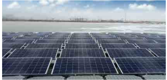
Datong Daqing • China extremely cold region Installed capacity : 300kW
