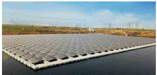
Huaiyang Zhoukou • China PV Poverty Alleviation Installed capacity : 200kW
